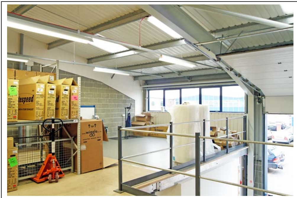
The installation of a two-tier longspan racking system, flooring and associated lighting and electrics as well as the installation of a mezzanine floor, which has doubled the area in the company's new 285 sq. metre facility.
